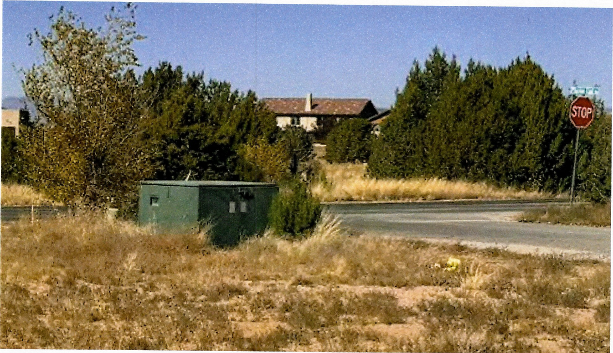
Power Transformer & Telco NW Corner of Parcel
